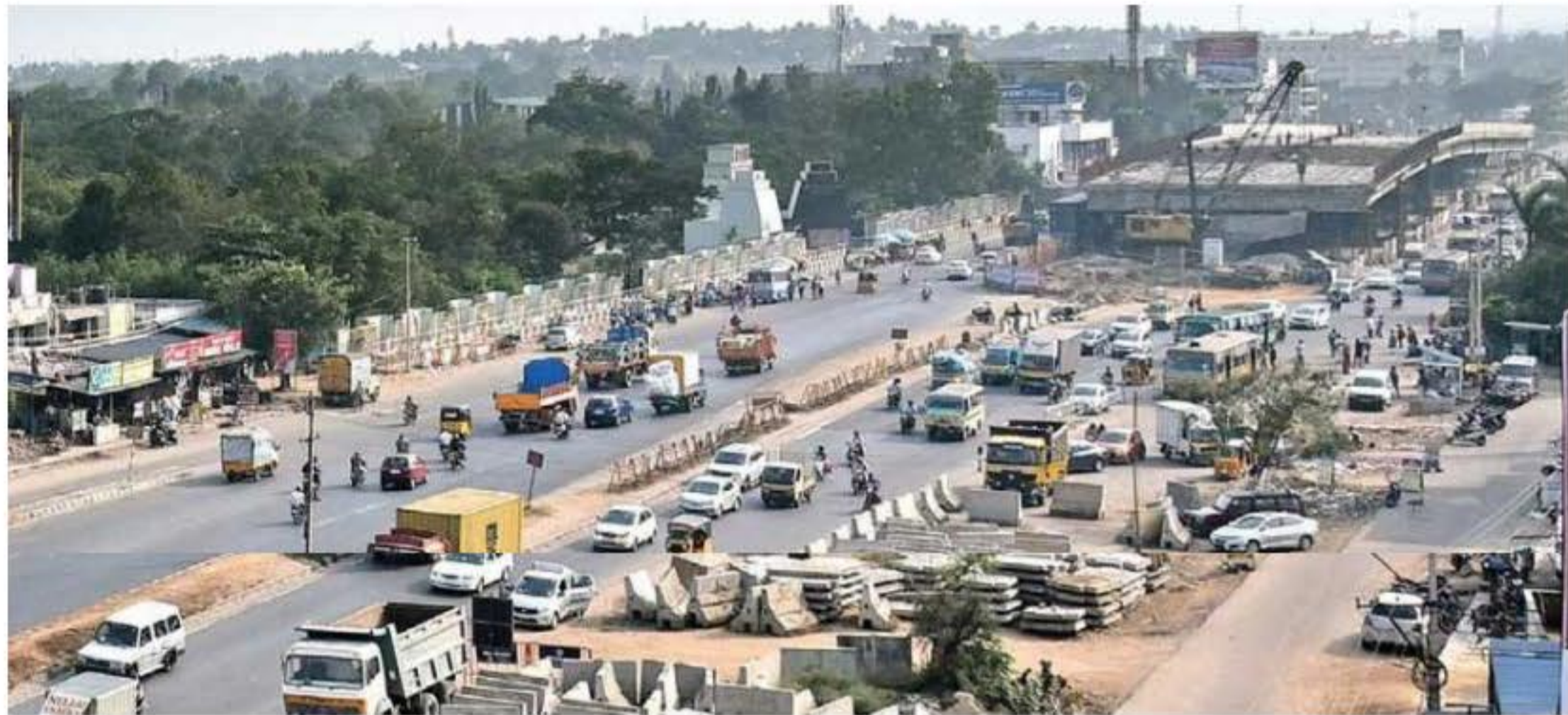
The Irumbaliyur-Vandalur stretch of Grand Southern Trunk road (NH 32) as seen on Monday | P JAWAHAR
